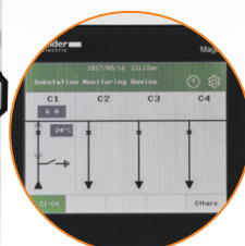
Substation monitoring device
